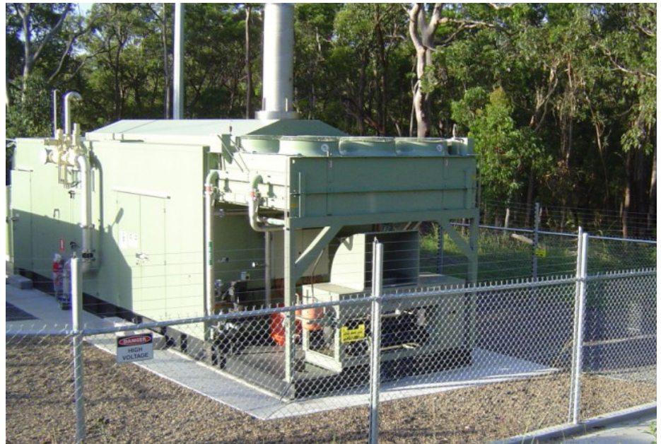
Awaba Renewable Energy Facility
